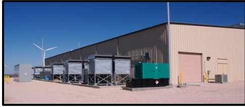
36 MW / 24 MWh Lithium Ion - West Texas
