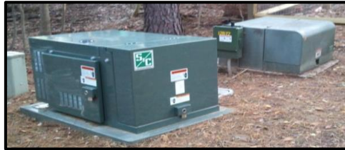
25 kW / 25 kWh Lithium Ion - Charlotte, NC
