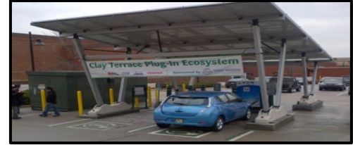
75 kW / 42 kWh Lithium Titanate - Indianapolis, IN (Carmel)
