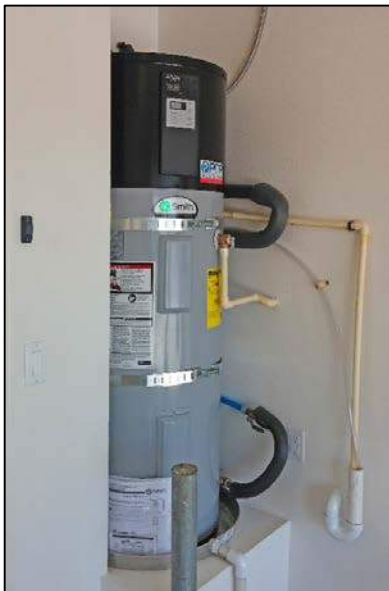
Electric Heating and Water Heating
